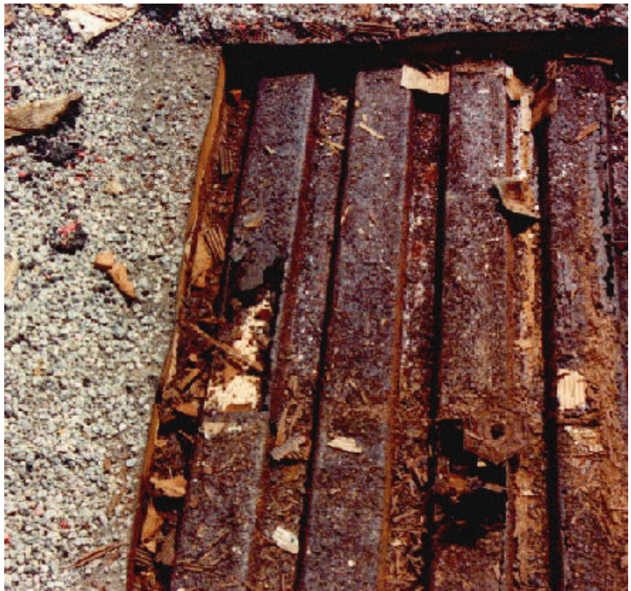
Figure 2: From Project No. 1, severe corrosion of deck, plate, and fastener.
