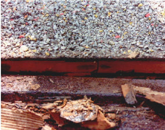
Figure 5: Project 1, view of wet insulation.
