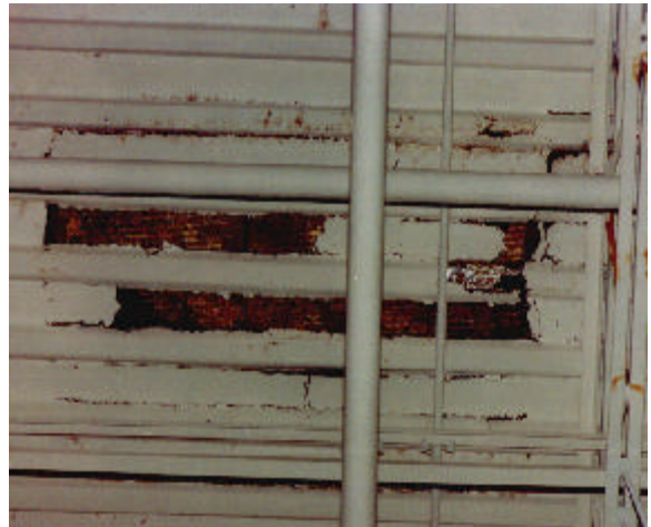
Figure 6: Project 1 interior view of corrosion
